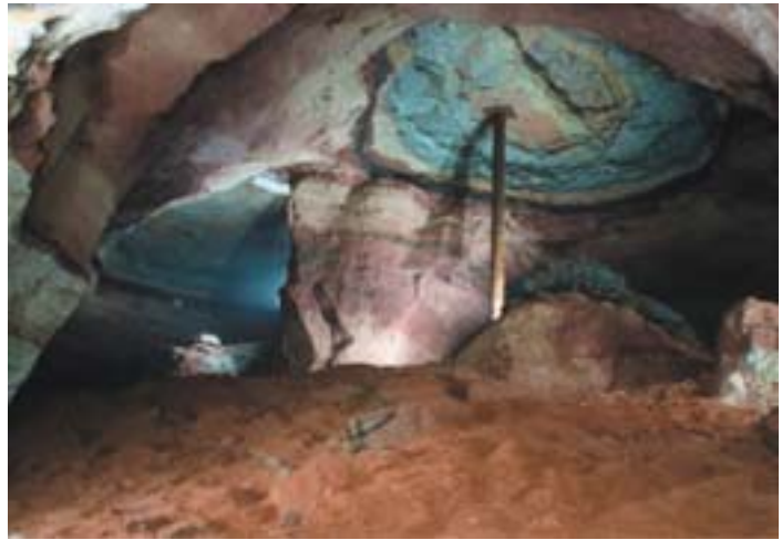
Fig. 13. Sablino Complex Monument. Levoberezhnaya Mine, the fastening of the unstable part of ceiling
