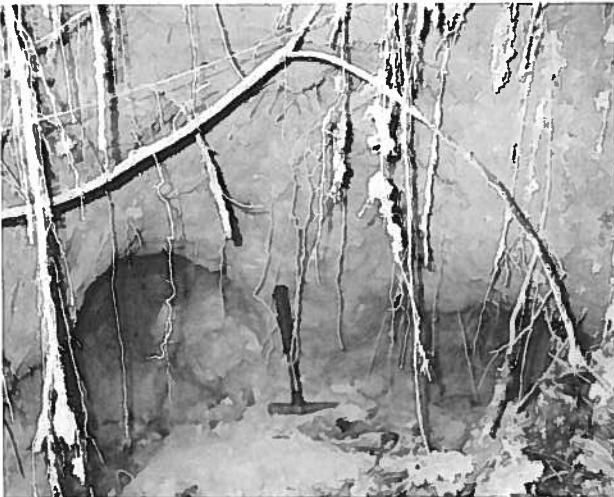
Fig. 2. Two branches of the western part of Tunnel in Bugaj in the middle (collapsed) entrance of the cave – state in March 2002.
